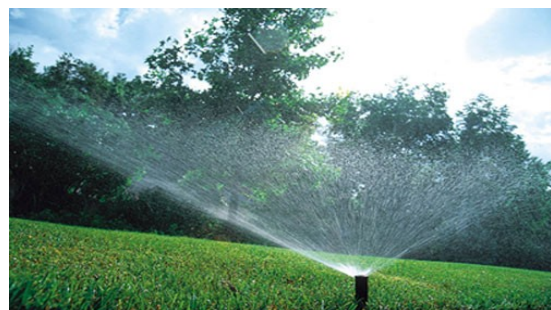
Sprinkling system in dryzone nursery
